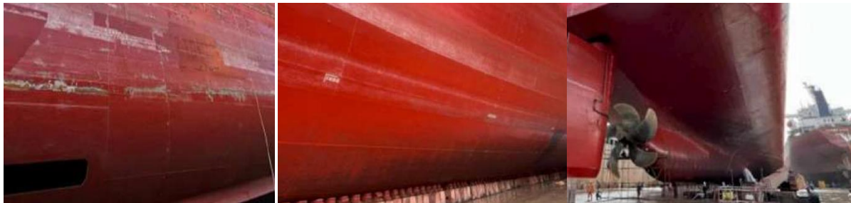
Fig.7b: Arrival condition in dock of container carrier after 62 months Hempaguard X7 application. No hull cleanings, 75% activity, 25°C water, 16 knots speed
