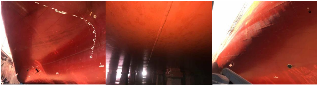
Fig.7a: Arrival condition of MR tanker with Hempaguard X7 and 50 months DD cycle. No hull cleanings, 55% activity 27° C water temp, 12 knots operational speed
